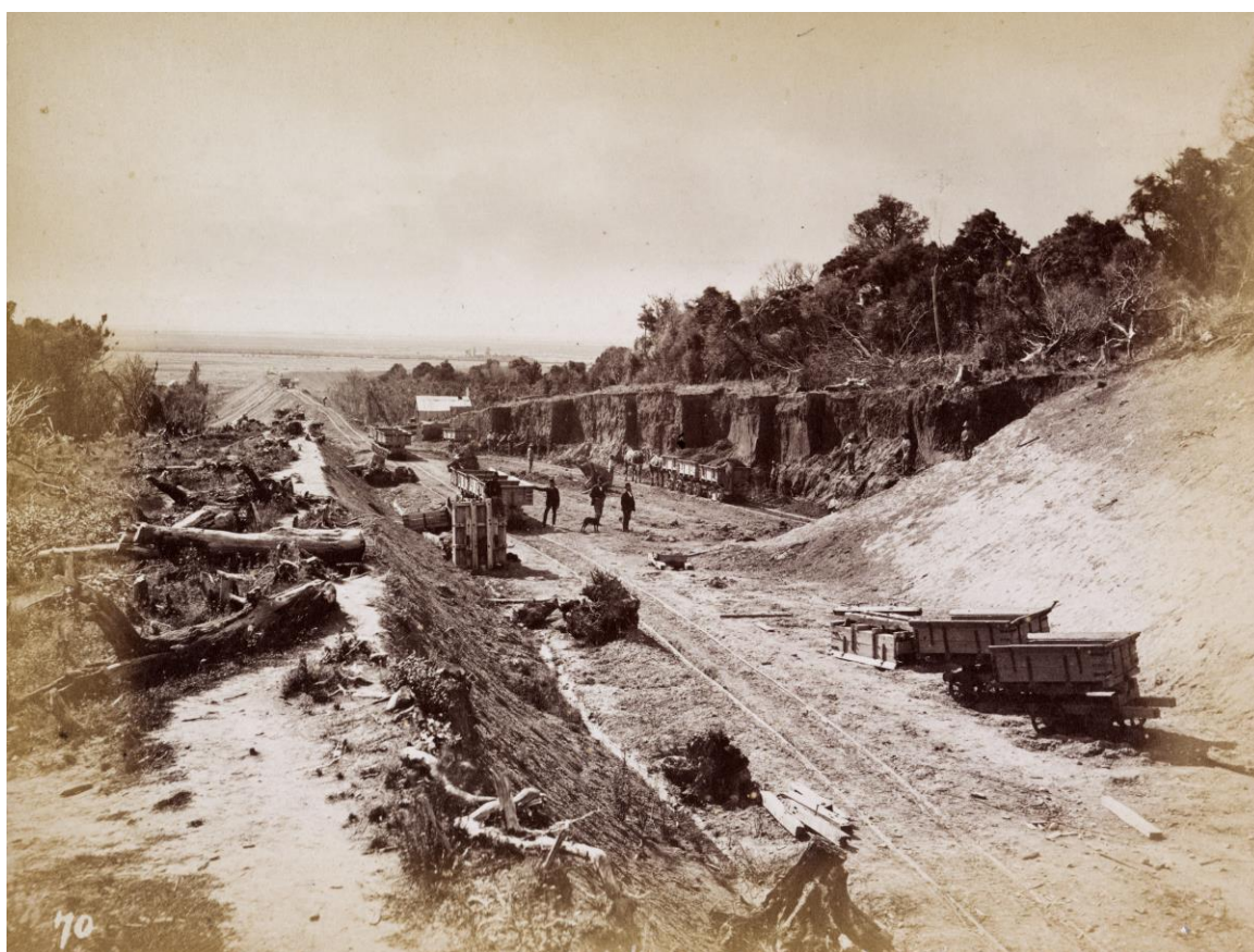
Figure 13: The Invercargill to Mataura line in 1874 at the north end of the Edendale cutting. Bush was cleared for a chain and half from the centre-line before the excavations could begin. The resulting timber was able to be used by the contractor for whatever purpose he desired. The pattern created by earth falls is seen in the middle-distance. The earth fall was a technique commonly used in South Island gold mining, where a face (or lift) of earth was undermined causing it to fall so it could then be cleared. Photograph. Invercargill and Mataura Railway, north end, Edendale cutting , n.d. Hocken Collections - Uare Taoka o Hākena, University of Otago.
