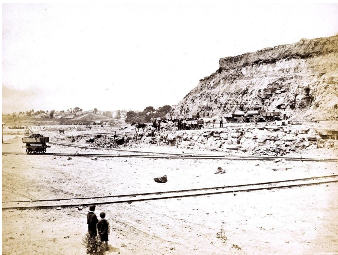
Figure 11: The Auckland-Drury railway under construction shows the scale of earth moving required for the preferred route for the line. The previous line was started following the discovery of coal. A large team of men are visible on the side of the cutting in addition to those with the horses and wagons. Photograph. Drury Railway, Auckland , n.d. Hocken Collections - Uare Taoka o Hākena, University of Otago.
