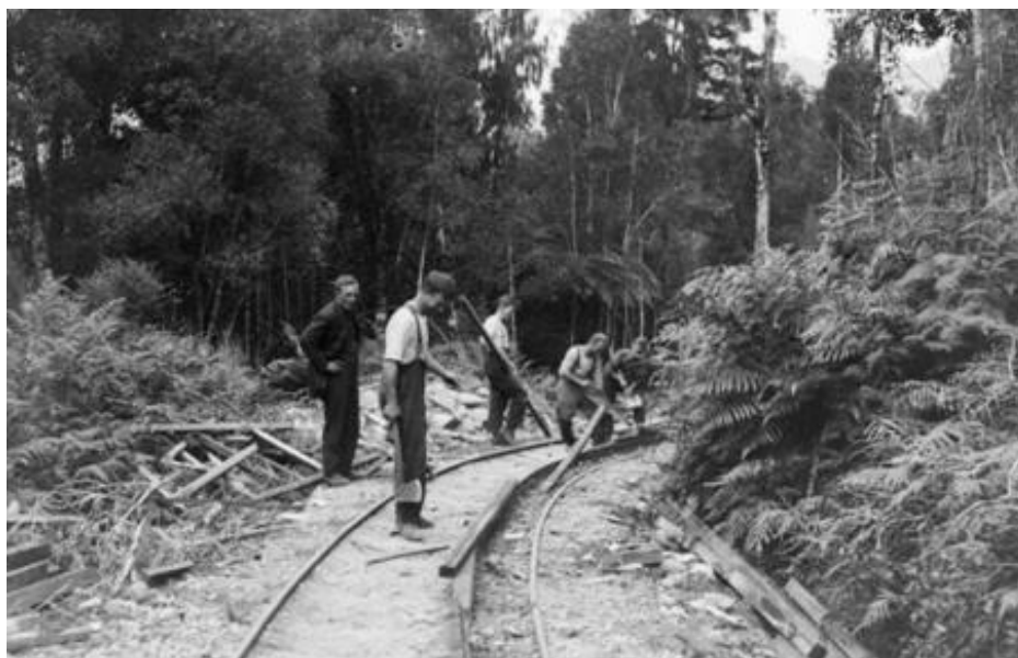
Figure 24: Labourers creating a curve in the railway line in Canterbury. Photograph. Railway construction workers working on tracks . Photographer unknown ( The Press ), Alexander Turnbull Library, Wellington, Ref: 1/2-041244-G /records/29946399
