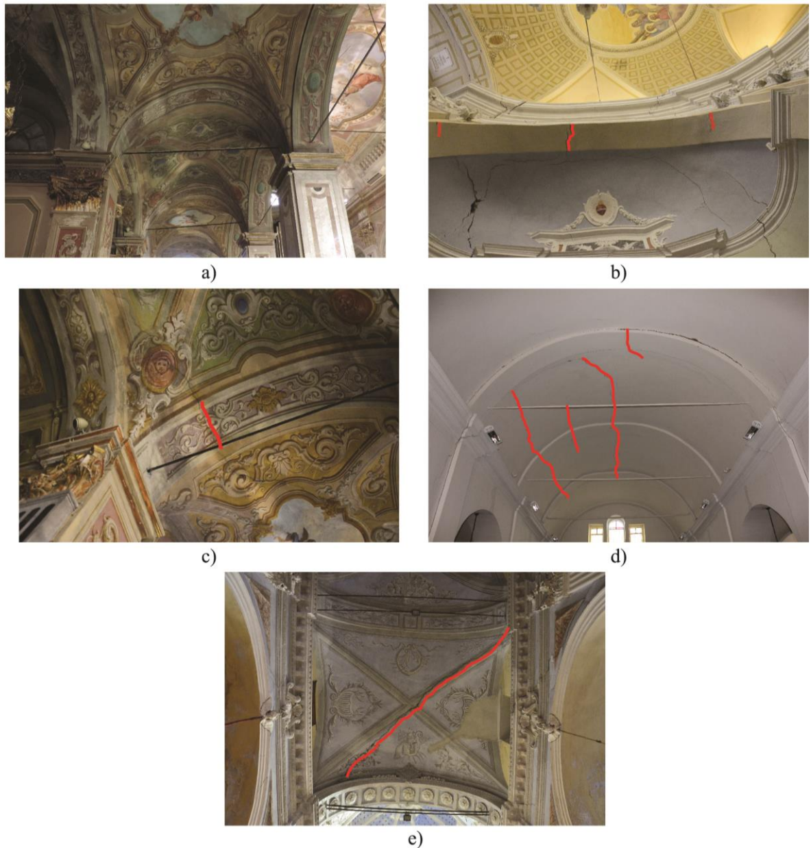
Figure 26 - Damage and deformation in arches and vaults a) large deformations (CH_13), b) symmetrical crack pattern (CH_4), c) asymmetrical crack pattern (CH_13), d) longitudinal cracks along the vaults (CH_22), e) diagonal cracks along one of the ribs in cross vaults (CH_22)
