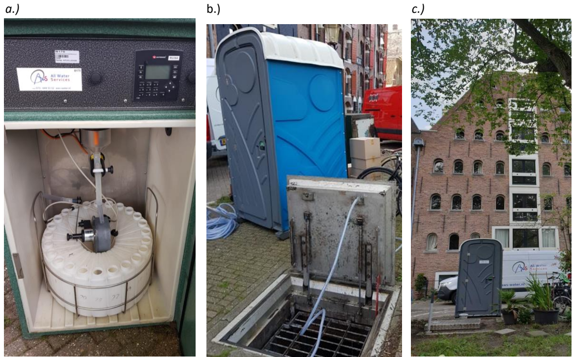
Figure 4.2-14. Photographs of wastewater sampling installation on Prinseneiland. From left to right, a.) Automatic sampling cabinet with 24 sample bottles, b.) Portable toilet that housed the sampling cabinet with sampling hose leading through the manhole cover to wet well below, c.) View of sampling location once the installation of the sampler was completed.
