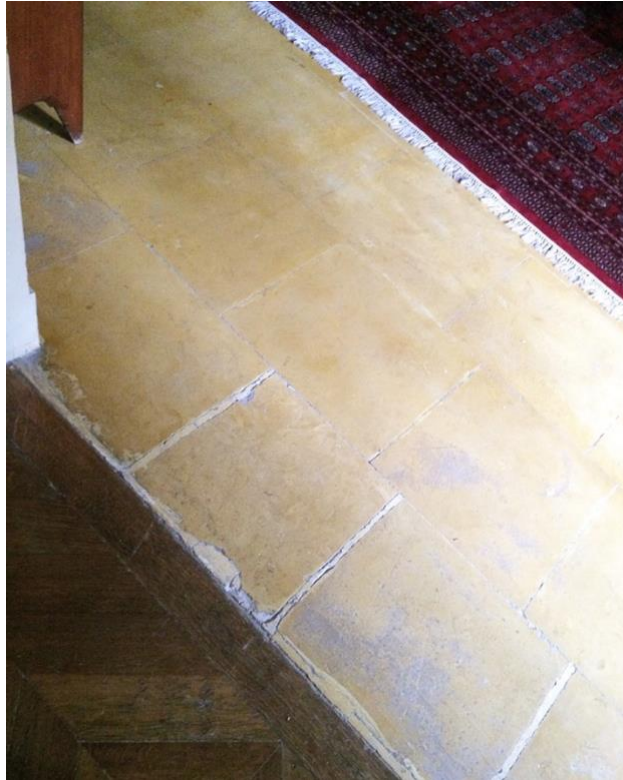
Figure 5.7: Floor finishes at San Anton Palace, ranging from original flagstone to parquet (Source: A Wismayer)
