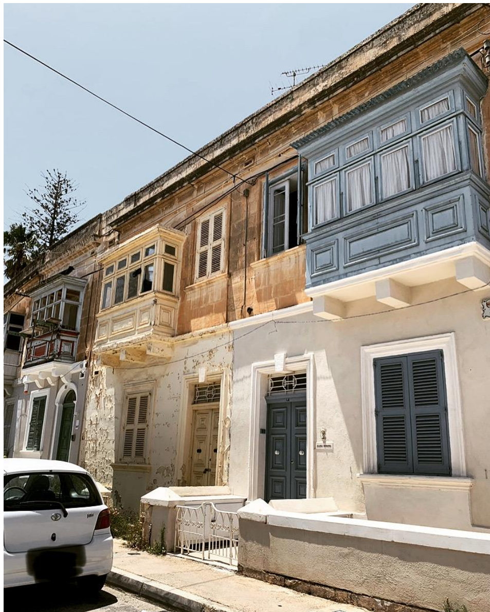
Figure 3.3: A streetscape of heritage building facades that (from left to right) are undergoing, require or have undergone restoration works (Source: A Wismayer)
