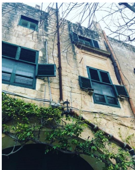
Figure 5.8: Timber apertures with louvres overlooking the private gardens, San Anton Palace (Source: A Wismayer)
