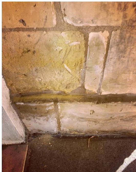
Figure 5.10: Powdering of limestone wall along the lower courses (Source: A Wismayer)
