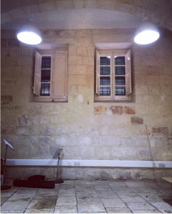
Figure 5.12: Lighting system for a converted office space, San Anton Palace (Source: A Wismayer)
