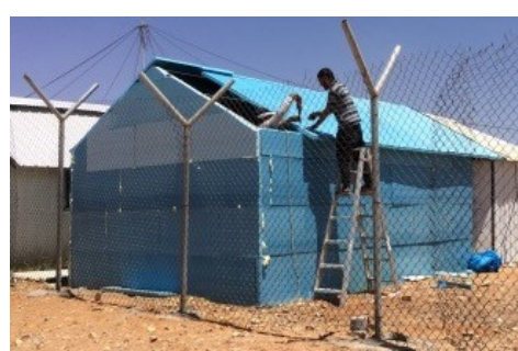
(h) XPS insulation and roof shade (ID 7; 40 mm insulation and roof shade with increased overhang)
