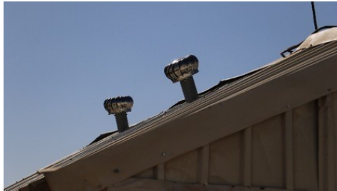
(c) Increased ventilation (ID 2; 4 high and low-level vents each and additional window)
