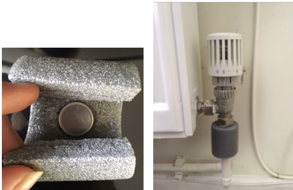
Figure 4.1: Preparation and placement of radiator sensor
