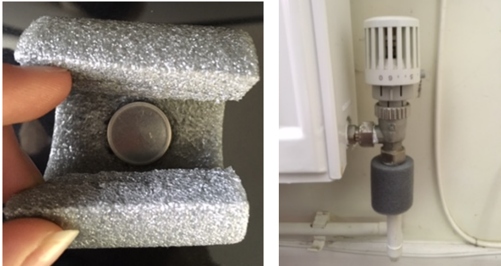
Figure 3.9: Method of attaching the radiator sensor to the radiator. Insulation pipe, cut to 5cm, with small indent for sensor to fit was taped around the pipework on the radiator.
