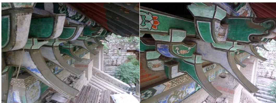
Figure 9 Original Dou-Gon sets on Qinghui Hall at Weiyuan Temple, Henan Province, China
