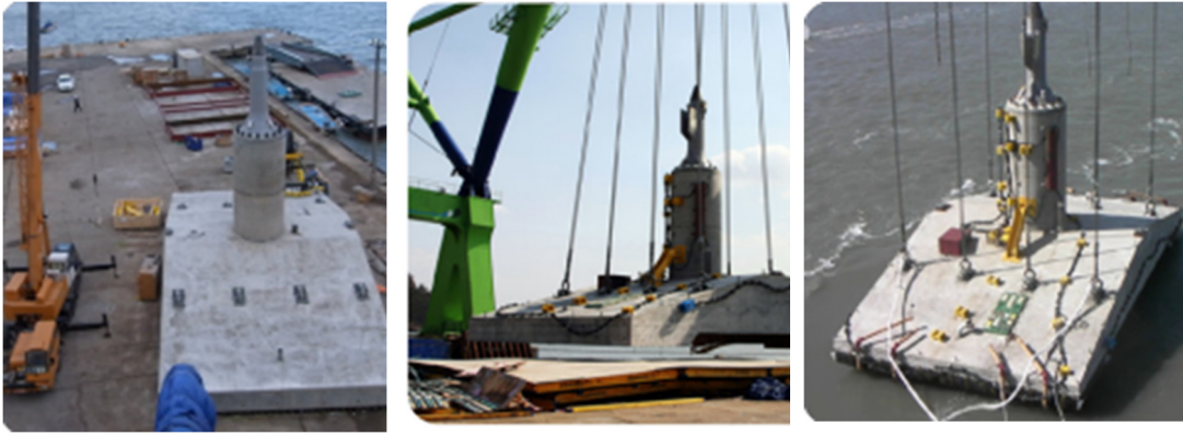
Figure 2-7. Voith Hydro Tidal Turbine's Concrete Gravity Foundation (Source: STRABAG Offshore Wind GmbH)
