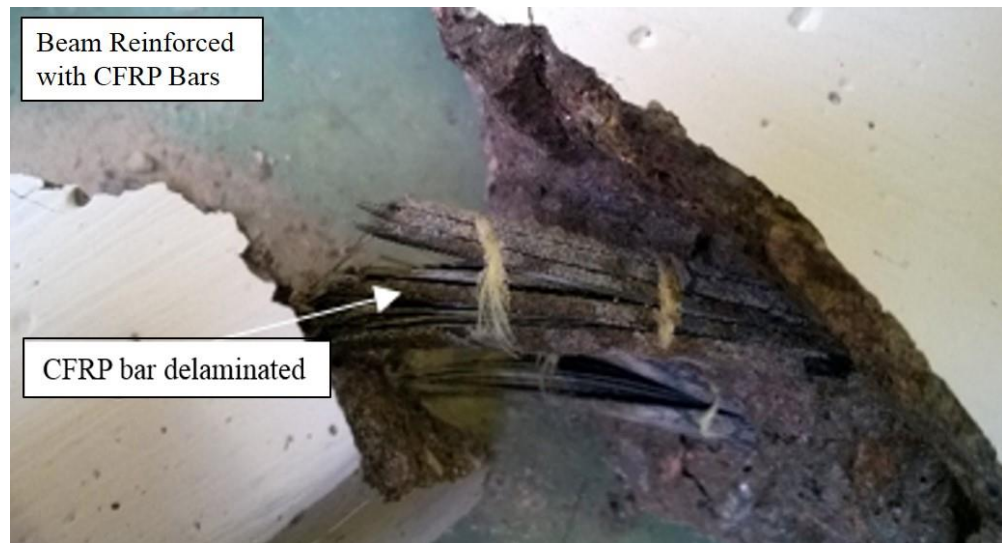
Figure 4.8 Rupture of the CFRP bar at cracked sections of the beam in the form of material delamination
