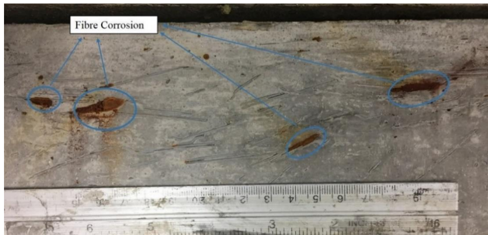
Figure 6.2 Minor corrosion of uncovered steel fibres at the bottom face of the beam
