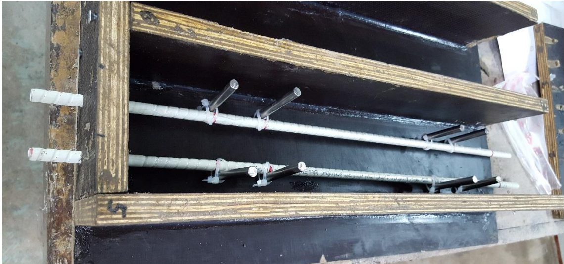
Figure 3.7 One FRP rebar cage with transverse CFRP bars tied on to longitudinal GFRP bars with the cable ties
