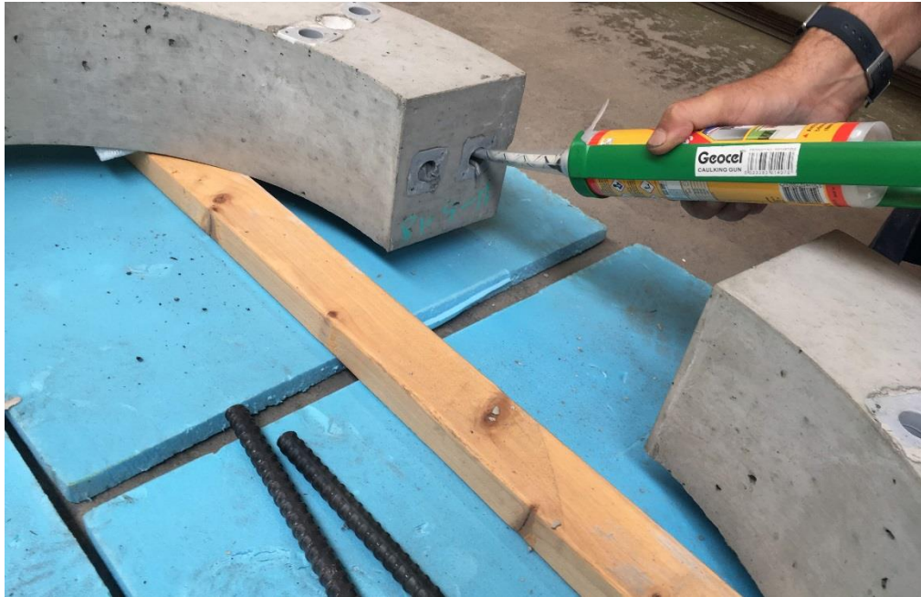
Figure 3.5 Injecting the AnchorFix ® -1 grout into the dowel connector sockets of the prototype ring component
