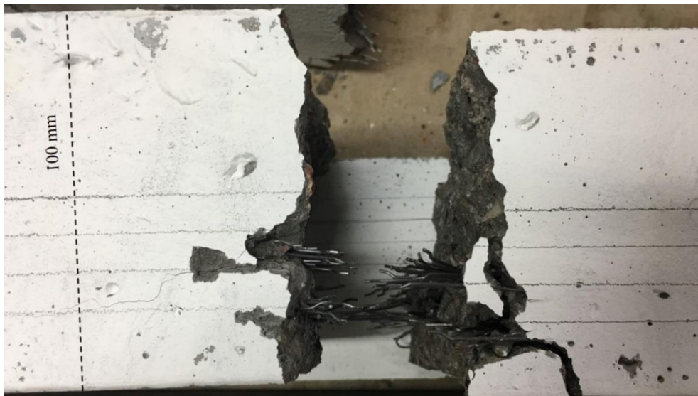
Figure 6.3 Aligned steel fibres at the cracked section of the beam after the bending
