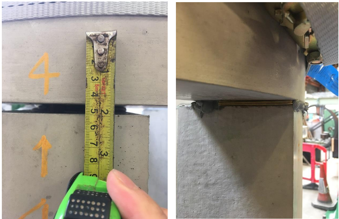
Figure 7.10 Gap between the longitudinal element and the middle ring (left), and filling the gap with thin steel plates (right)
