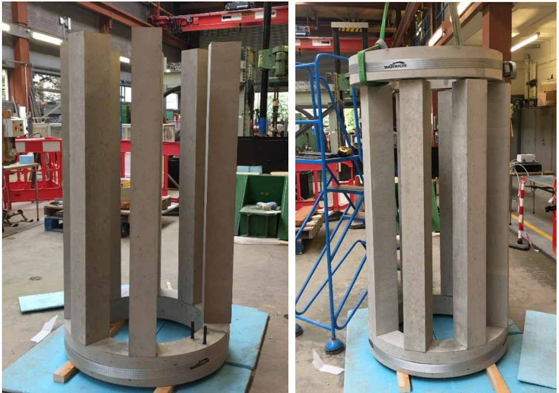
Figure 7.8 Assembly of the longitudinal elements on to the ring section vertically (left) and the middle ring on to the erected longitudinal elements (right)
