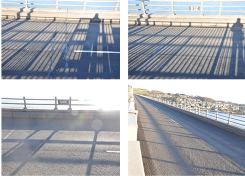
Figure 7-18 Abnormal expansion joint style of No. 30, 31, 32, 33
