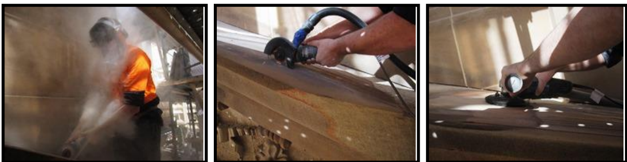
Figure 4: 'Chopping out' no dust shroud, Figure 5: 'Chopping out' with dust shroud, Figure 6: 'Spinning' with shroud
