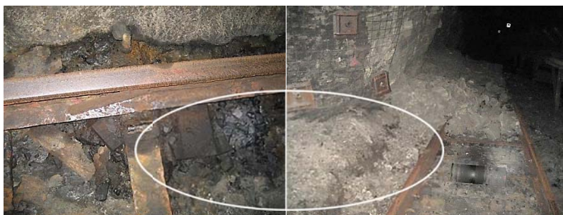
Figure 9: Damage to dolly-car rail & spalling in the conveyor drift
