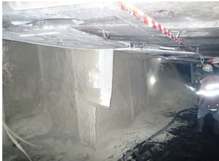
Figure 9: Shuttering off the fall material in preparation for consolidation of the muck pile and backfilling of the void in the roof
