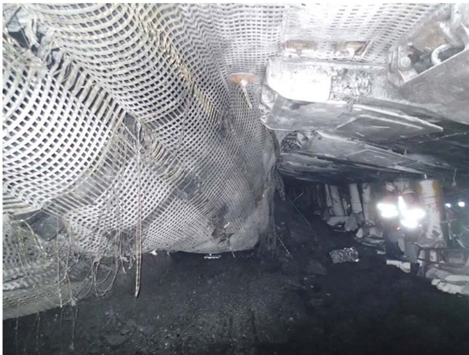
Figure 4: Fall of ground from shield 55 looking towards the E-frame
