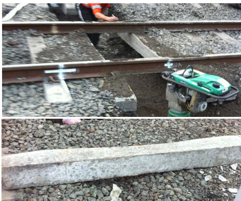
Figure 14: Abraded sleeper soffit (location adjacent to the test site)
