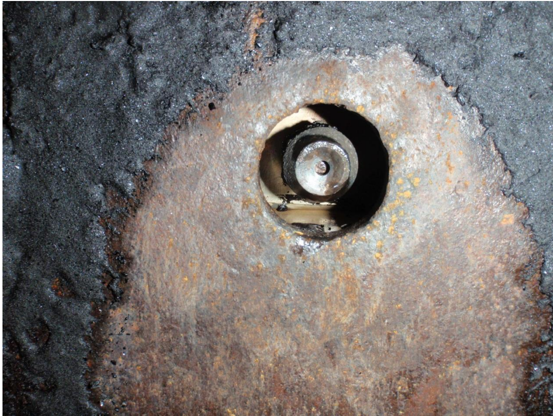
Figure 7.12 Mine A Spray Inside Discharge Hood
