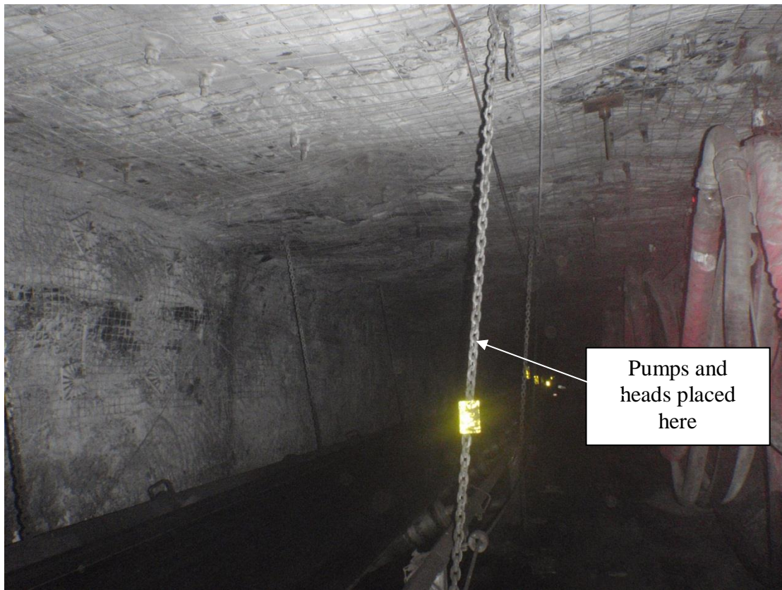
Figure 7.3 Mine A Pump and Head Location in the Belt Road
