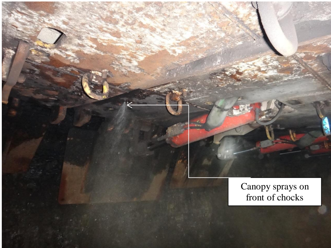
Figure 7.68 Mine E Installed Chock Sprays
