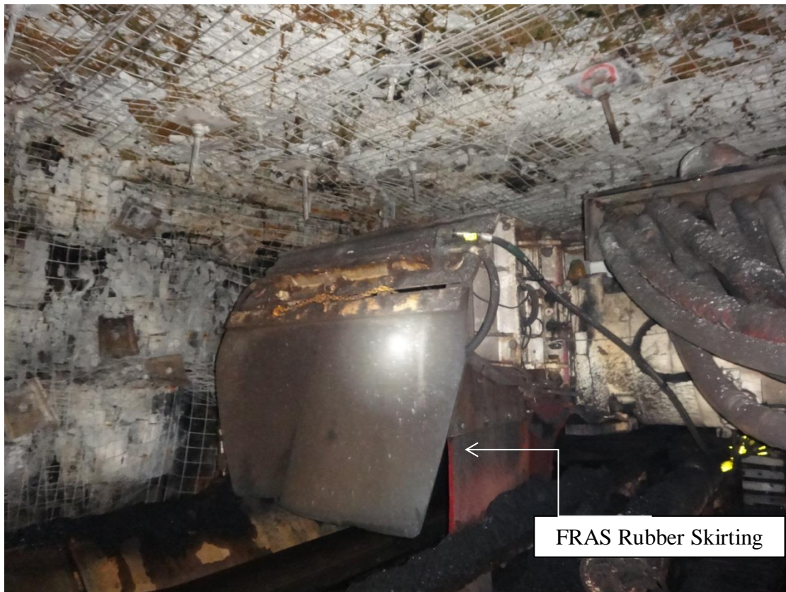
Figure 7.62 Mine E BSL Discharge Skirting
