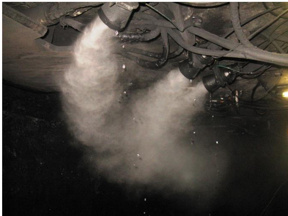
Figure 4.17 Venturi Sprays Installed at Chock # 5.
