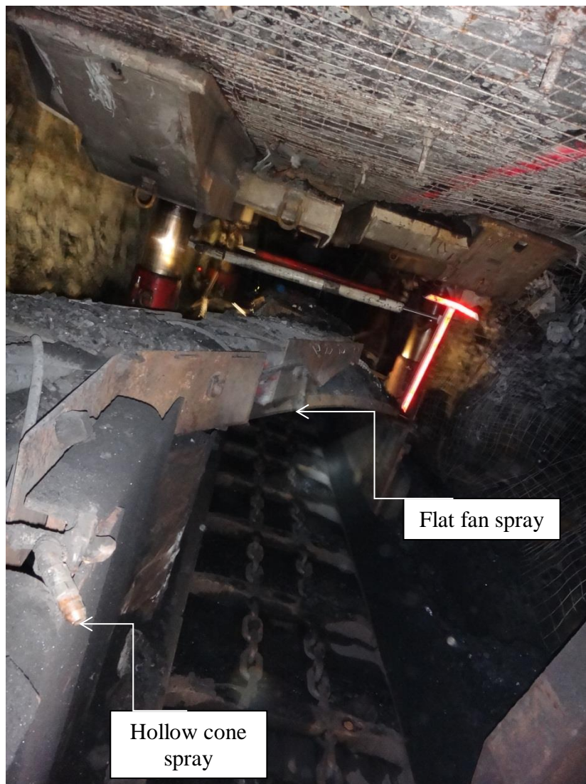
Figure 7.64 Mine E Crusher Intake Sprays
