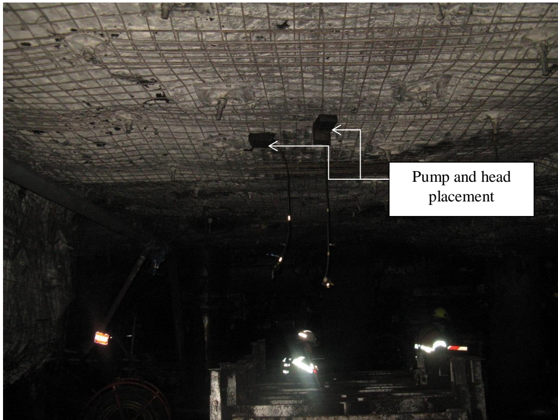
Figure 6.3 Pumps and Heads Positioned in LOC
