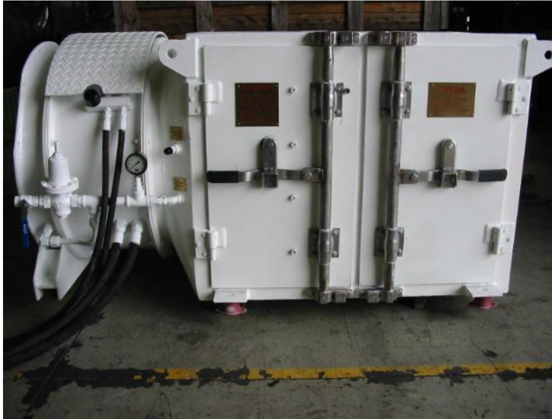
Figure 7.50 Mine C Installed BSL Scrubber
