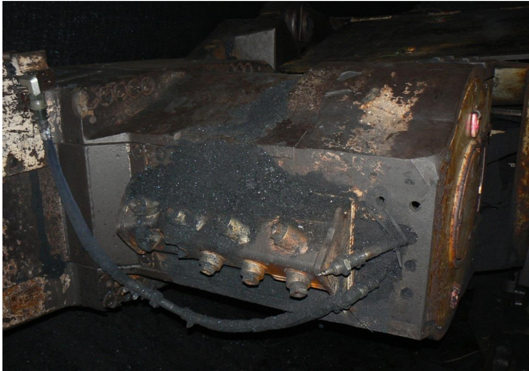
Figure 4.12 Spray Manifold Positioned on the Maingate Arm
