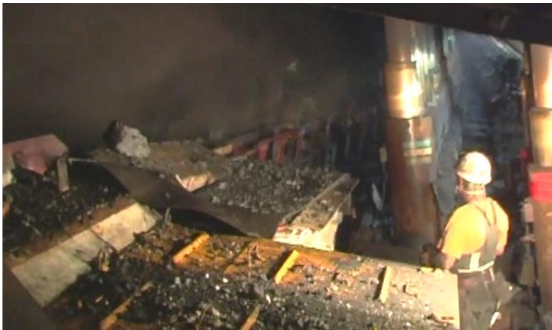
Figure 3.8 Dust Entrained into Walkway from Drum Cutting Floor
