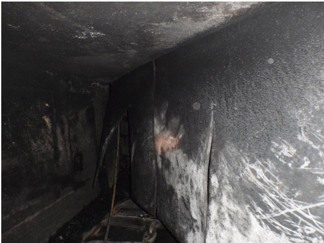
Figure 4.1 Conveyor Belt on the Intake to the Crusher
