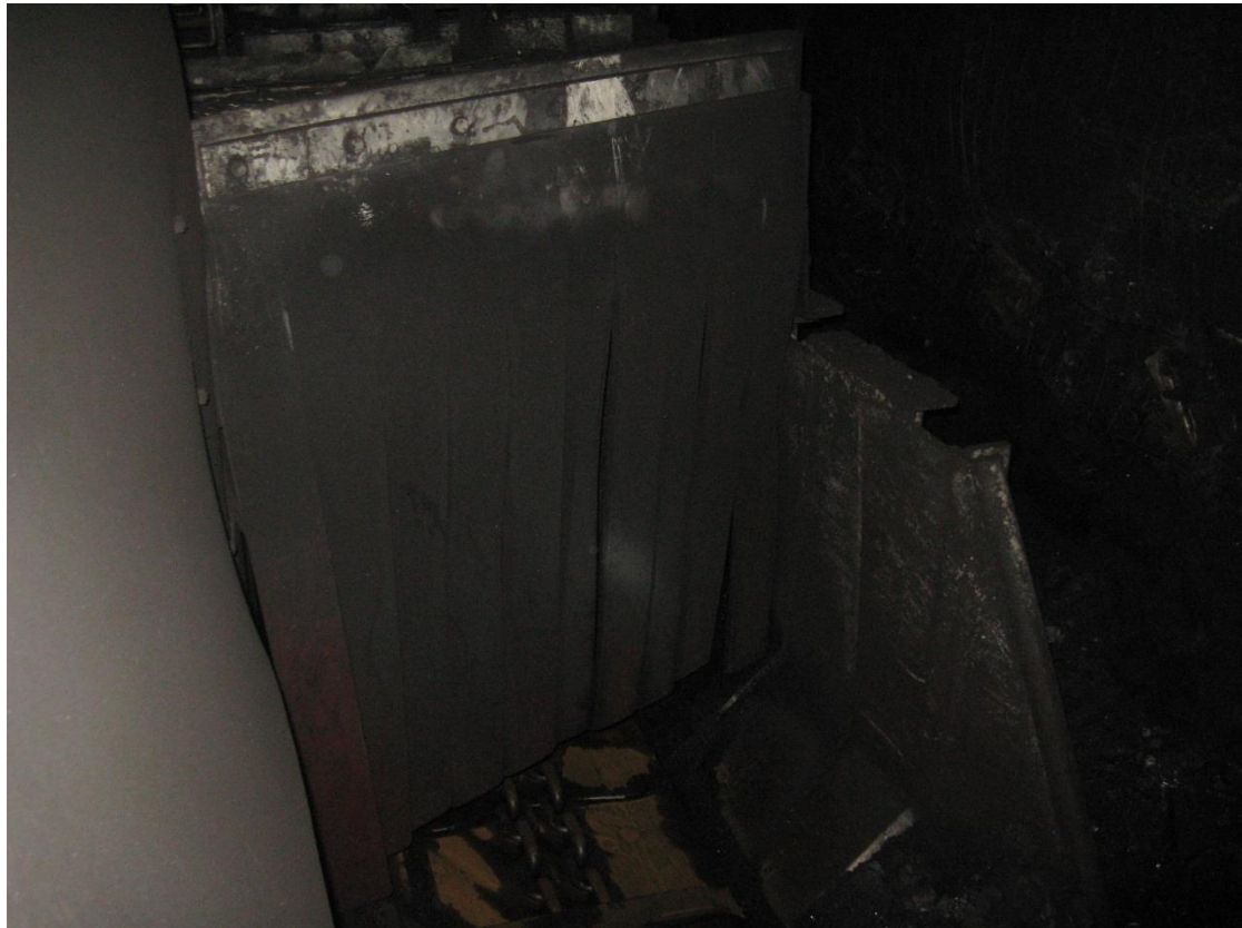
Figure 7.32 Mine B Rubber Skirting at Intake to Crusher
