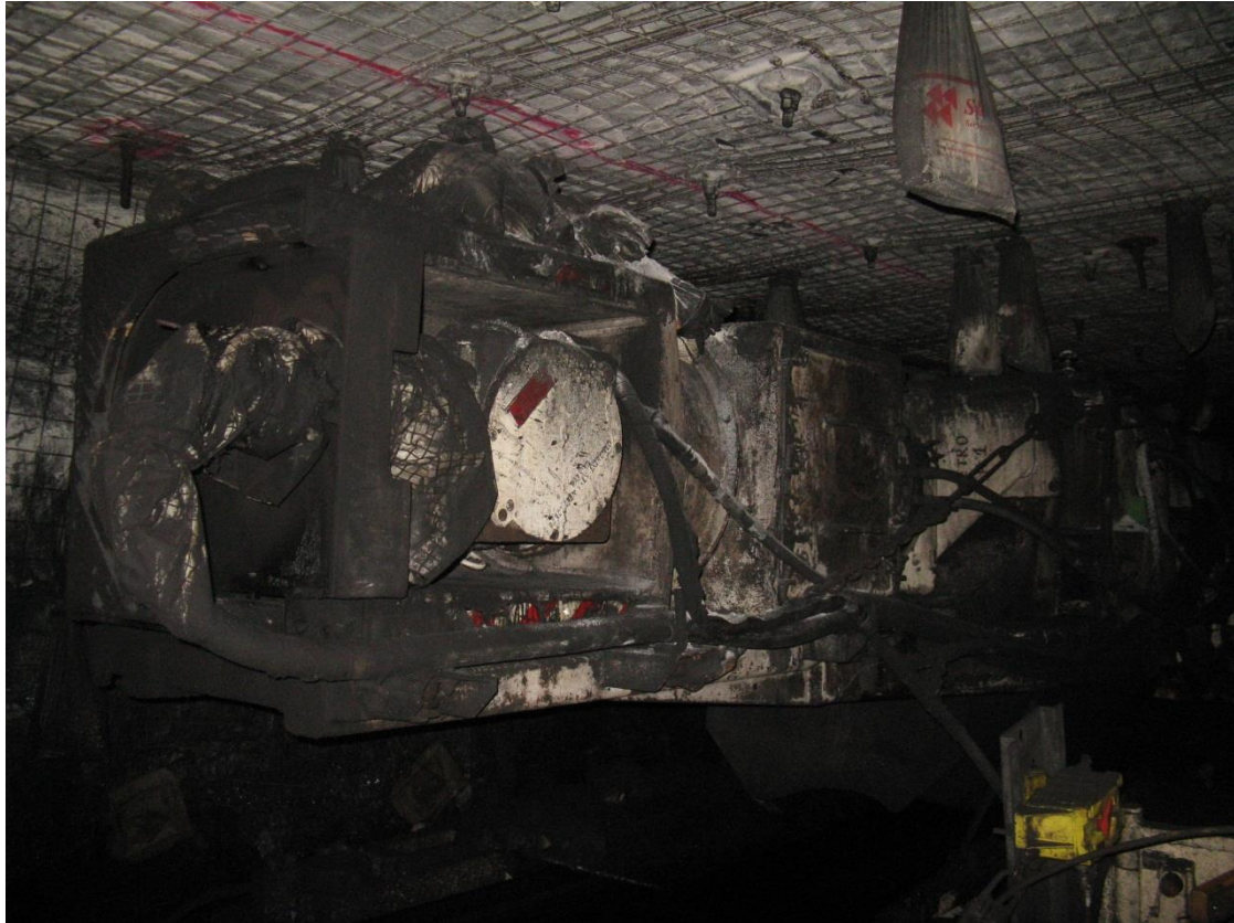
Figure 7.40 Mine B Installed BSL Scrubber
