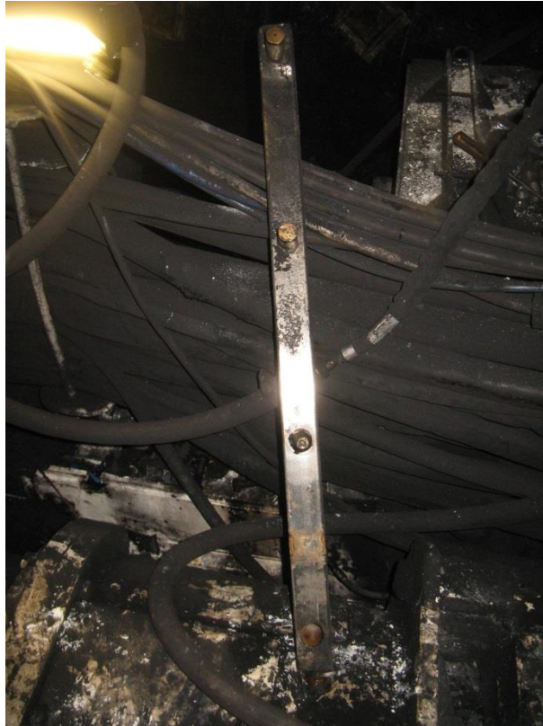
Figure 7.33 Mine B Installed Sprays in Spray Bar in Crusher
