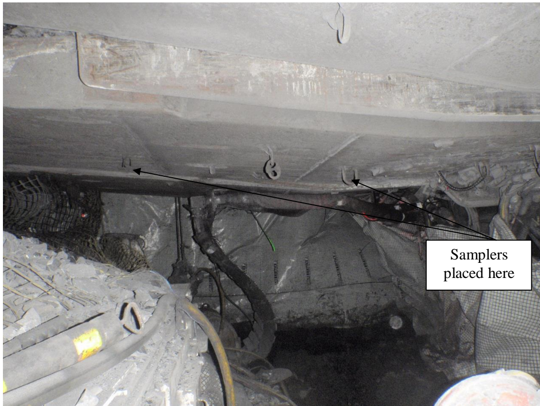
Figure 7.7 Mine A Pump and Head Location for Inadequate Crusher and BSL Sealing
