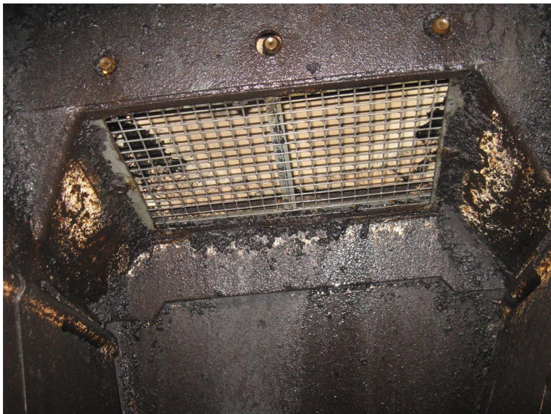
Figure 7.31 Mine B Sprays inside Discharge Hood
