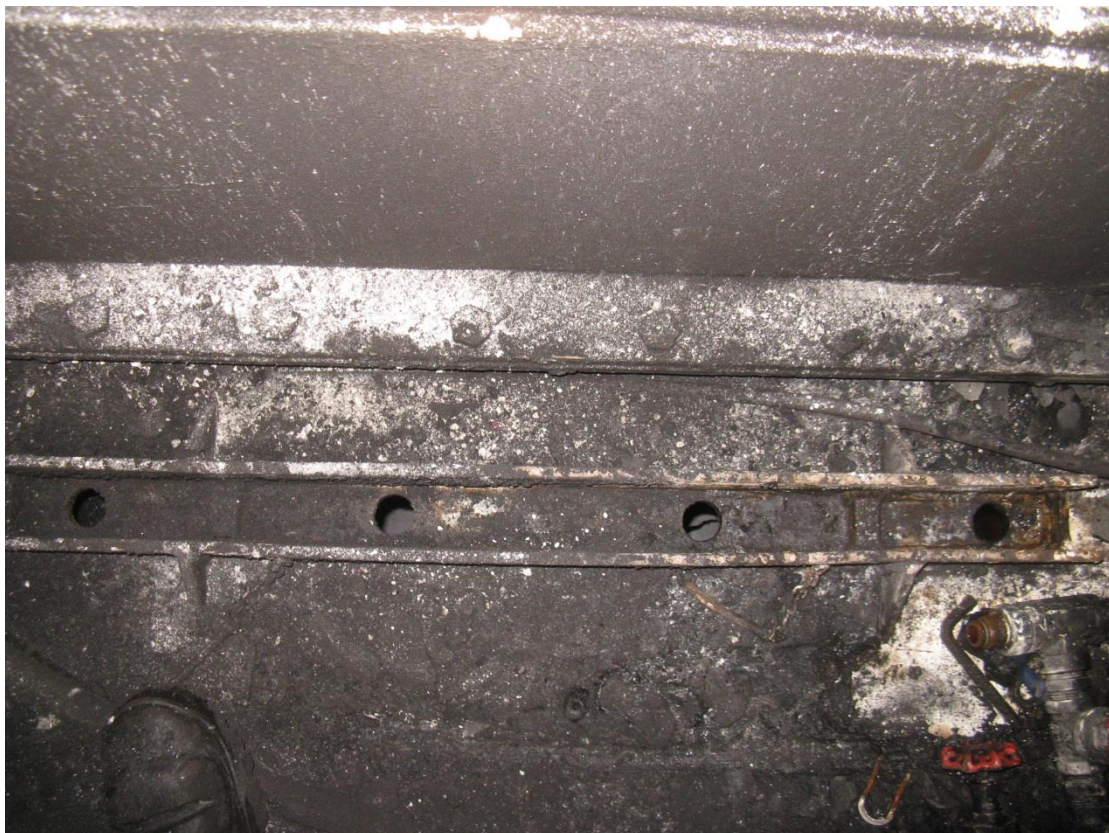
Figure 7.34 Mine B Spray Bar Location Holes in Crusher
