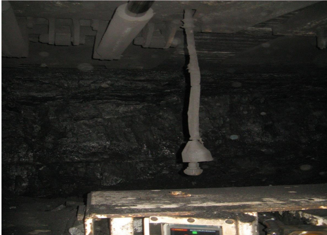
Figure 7.38 Mine B Dropper Spray at Chock #5
