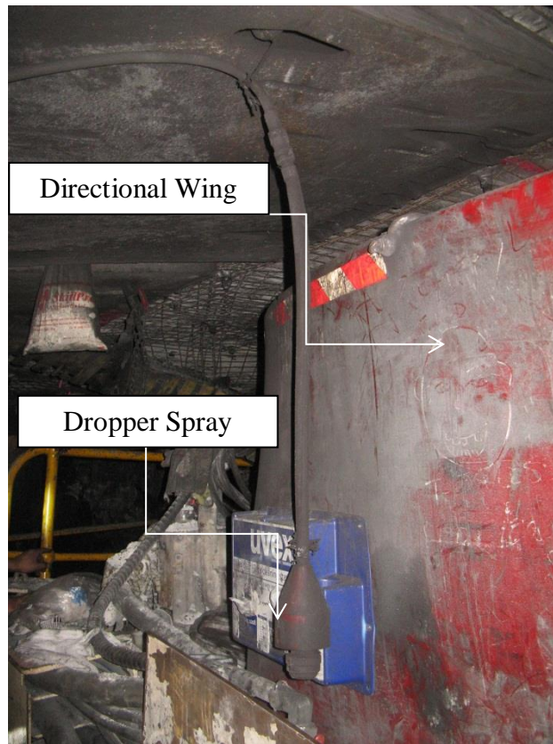
Figure 7.36 Mine B Dropper Spray at Maingate and Directional Wing
