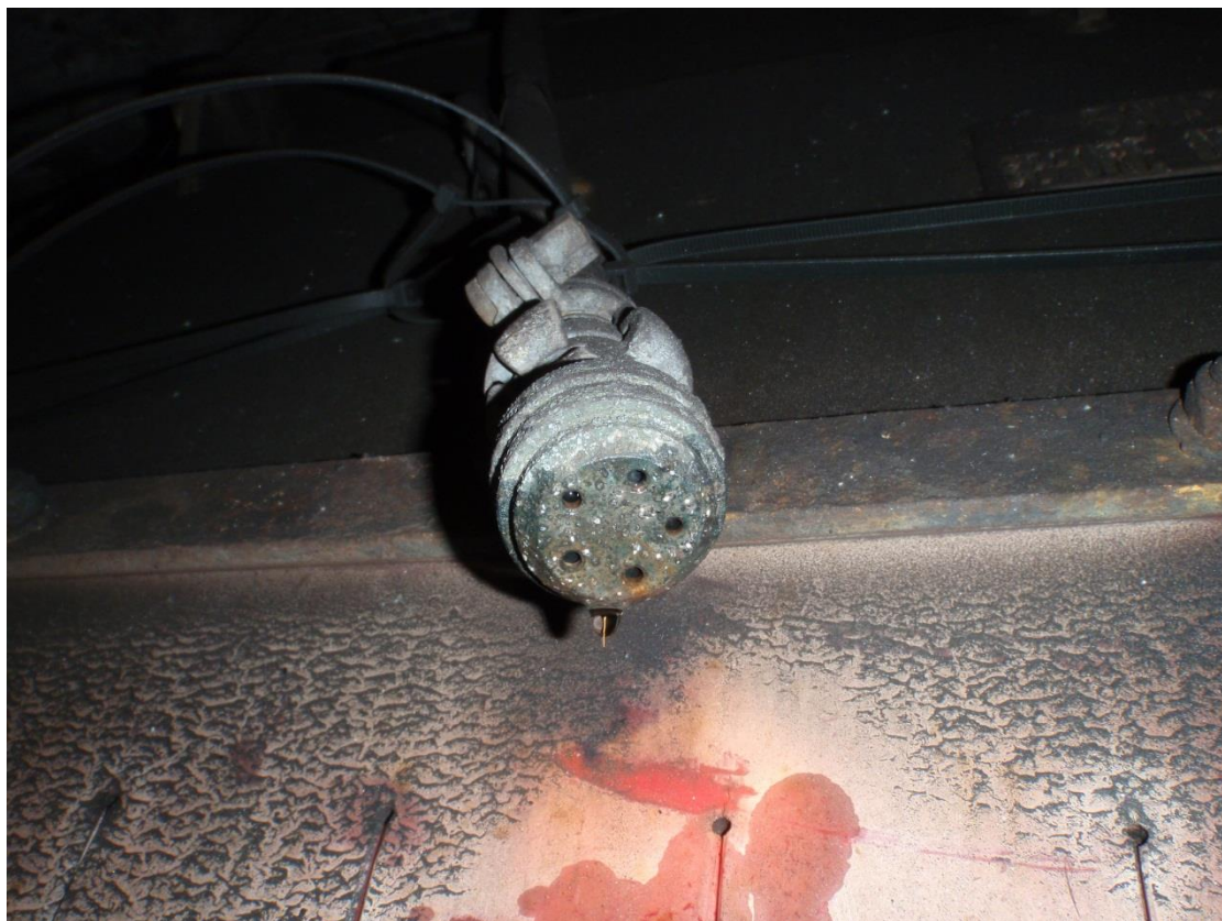
Figure 7.11 Mine A Code 96 Cluster Spray
