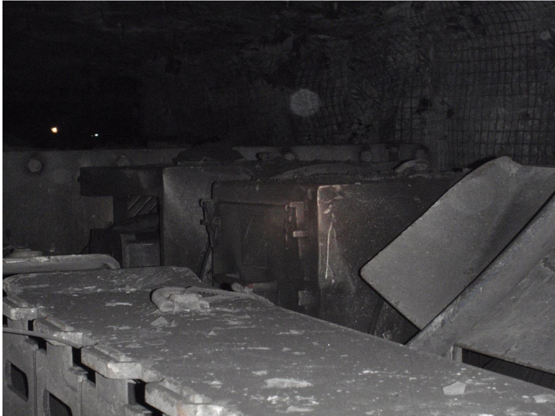
Figure 7.17 Mine A Installed BSL Scrubber
