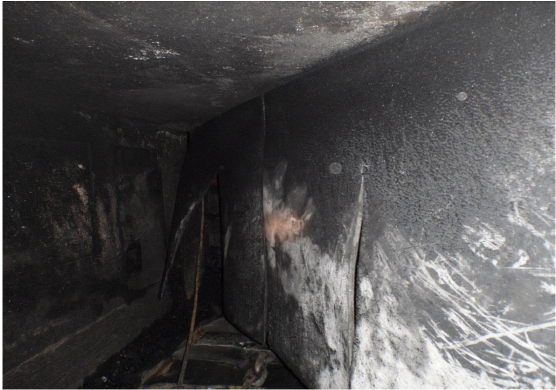
Figure 7.13 Mine A Rubber Skirting at Intake to Crusher
