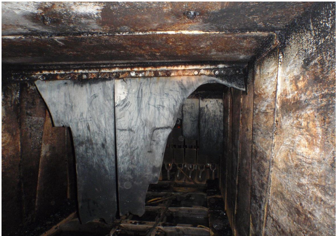
Figure 7.14 Mine A Rubber Strips Before Crusher
