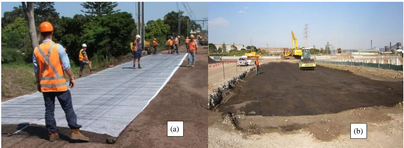
Fig. 1 (a) Installation of geocomposite at Bulli (b) Compaction of granular waste at Port Kembla
