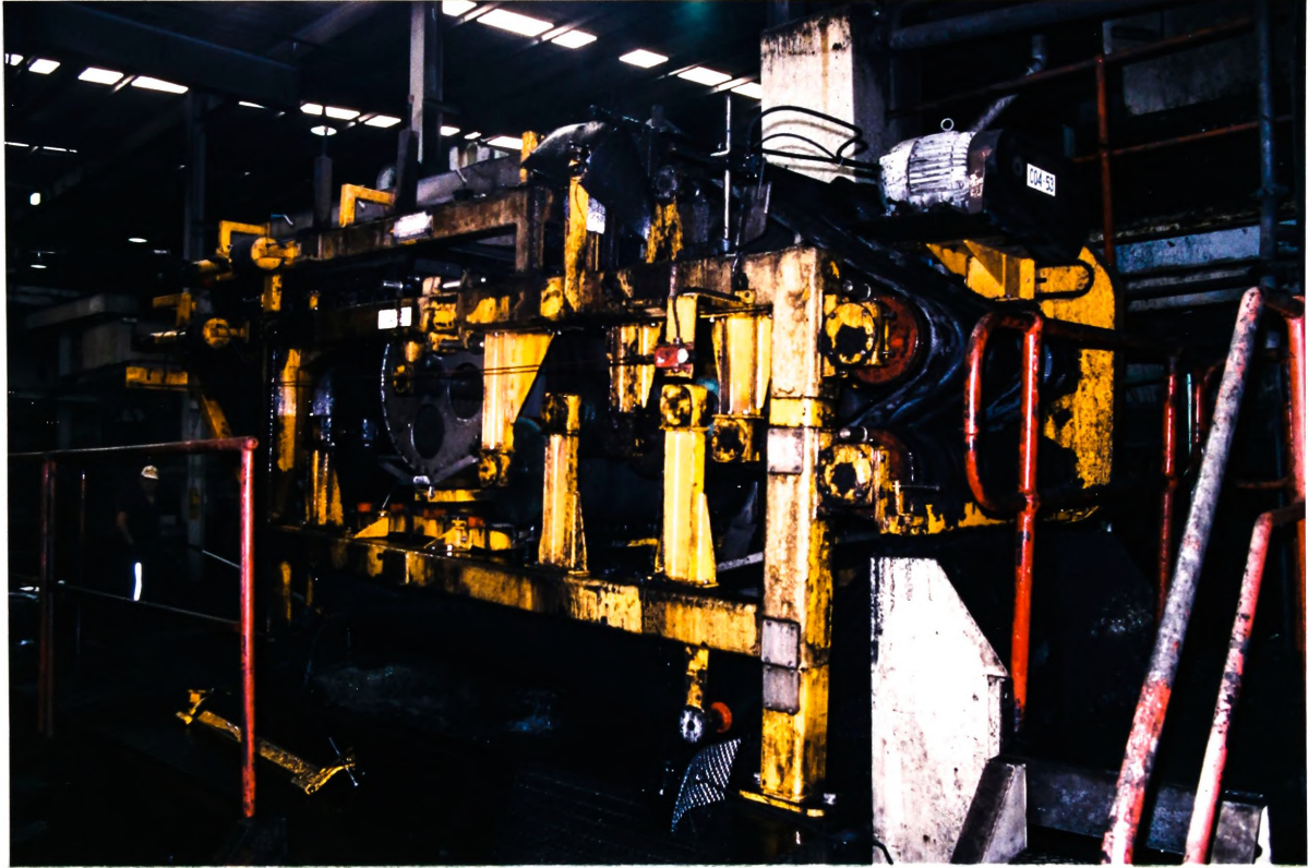
Figure 2.5: Band Press Filter, Used for De-watering of Slimes, in Operation
