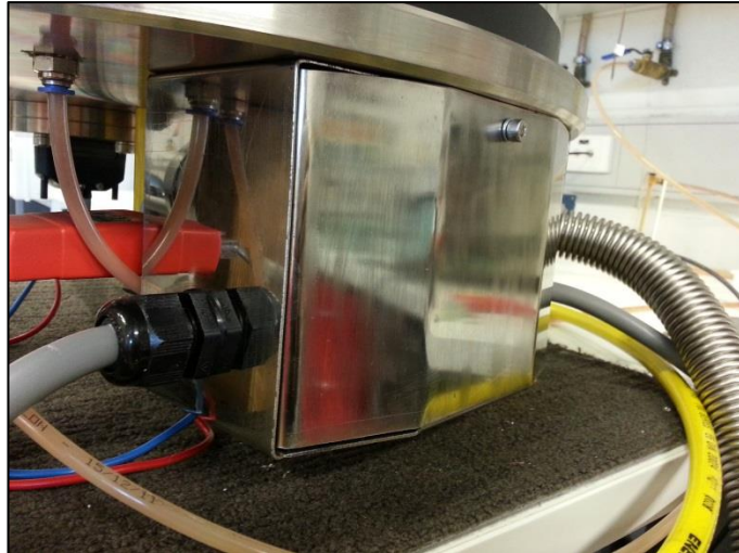
Figure 3.24. High power electrical feedthrough enclosure added for improved safety.
