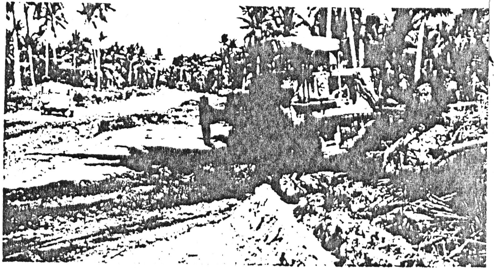
Widening road as part of 'upgrading' program to provide rural access to markets.
