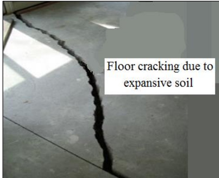
Figure 1.3: Cracked floor of a building founded on expansive soil (© of Arredondo Group)
