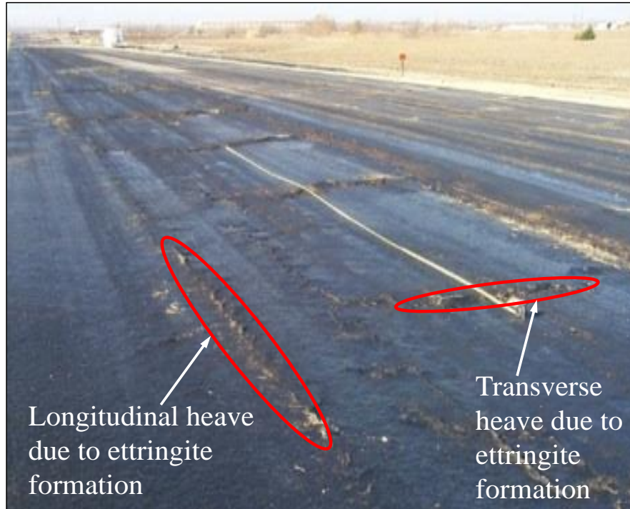
Figure 2.28: Vertical heave due to ettringite formation in sulphate bearing soil treated with cement in Texas, USA (After Harris et al. 2006)
