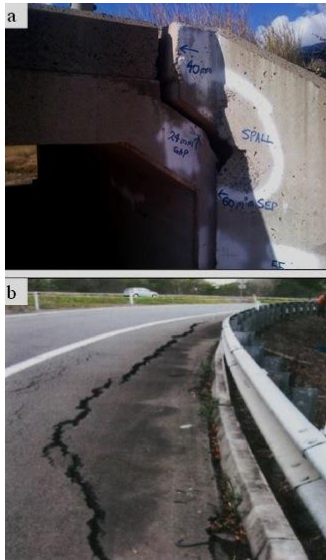
Figure 1.2 a): Cracked culvert wing wall of the drainage structure over Jingi Jingi Creek due to shrink-swell of the foundation soil on the Warrego Highway west of Brisbane, b): Longitudinal cracking due to expansive embankment material on the Cooroy exit off ramp, on the Bruce Highway north of Brisbane (© Queensland Department of Main Roads)
