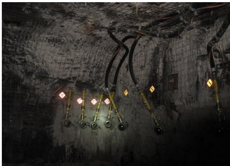
Figure 5.8: Field observation of gas drainage borehole location
