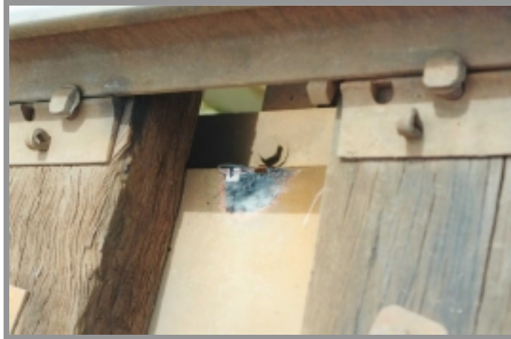
Figure 3.3.3. Strain gauge located on the top flange of the Broad Flange Beams above one of the web-stiffeners.
