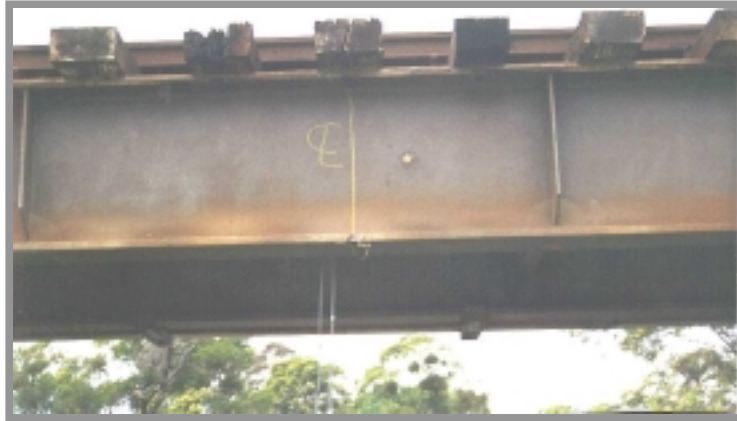
Figure 3.1.5. Broad Flange Beam with web-stiffeners welded on the top flange and web.
