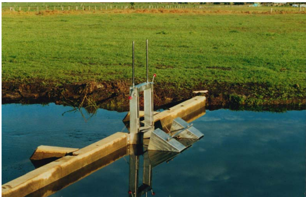
Figure 2.6 A self-regulating tilting weir (built in 2001 by the UOW ASS research team)
