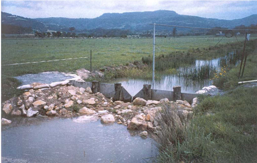
Figure 2.5 V-notch weir installed near Berry, south east NSW, Australia (Blunden, 2000)
