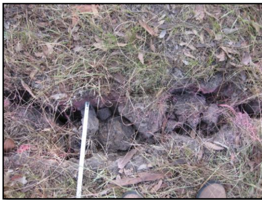
Figure 18 - Typical tension crack above total extraction panels with cover depths of 60-80 m
