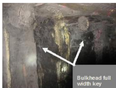
Figure 6 - Bulkhead 300 mm depth key with Tensar mesh removed and PUR injection of a central ring of holes
