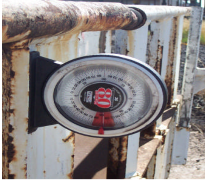
Fig 17 – Magnetic Inclinometer attached to Bretby. Panline LW103
