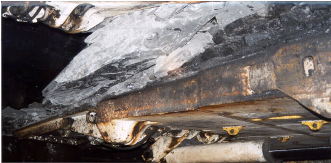
Fig 13 – Open cavity above the gate end supports at the maingate LW102
