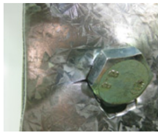
(a) Punching failure
