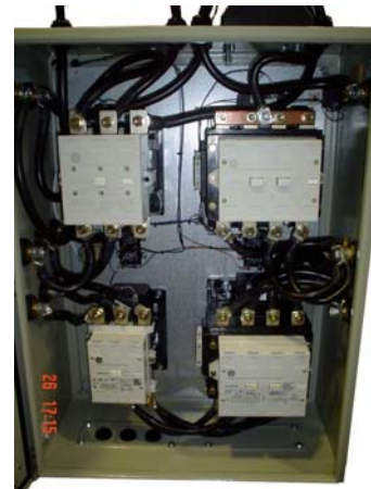
Figure 6. Test System Contactor Enclosure
