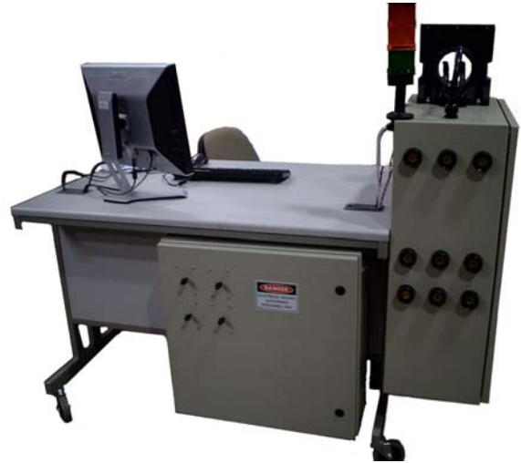
Figure 4. Test System Control Centre
