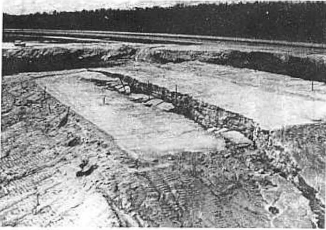
FIG. 2. View of Tensile Fracture of Compacted Fill
