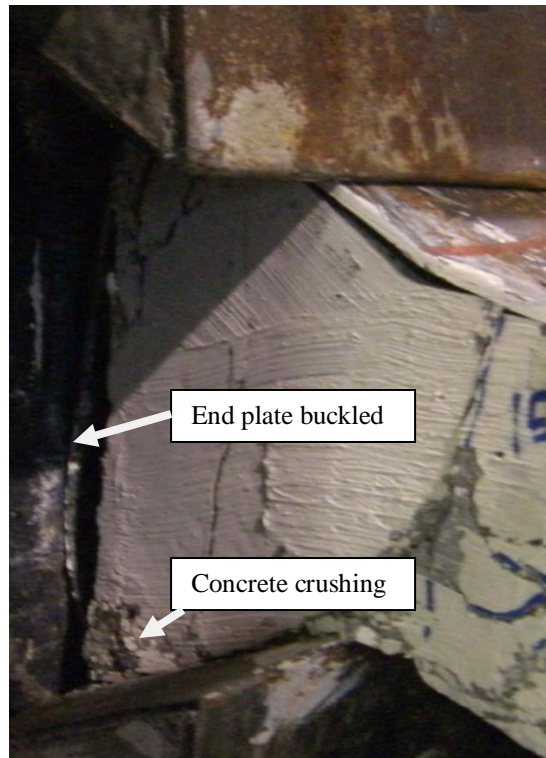
Figure 5.30: Crushing of lightweight concrete and buckling of steel end plate for the Lightweight core panel.
