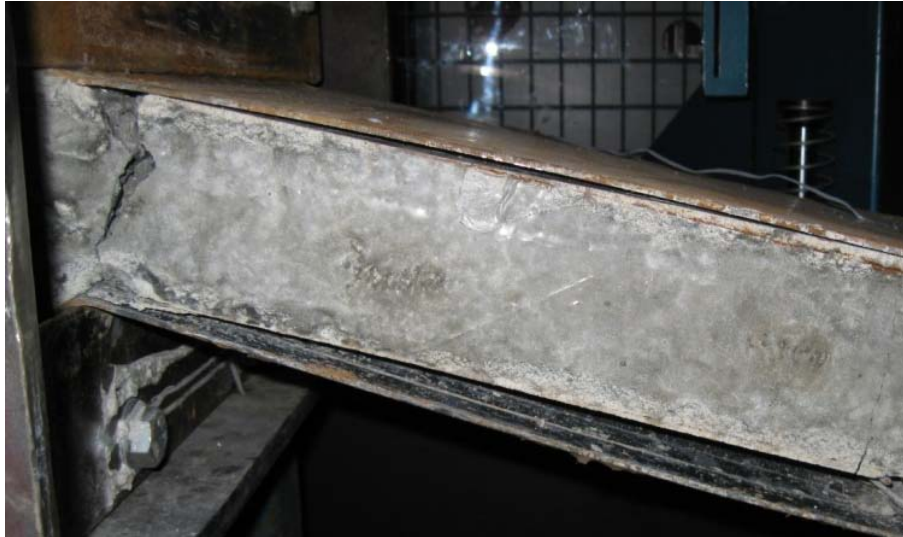
Figure 7.26: Separation of wire meshes from the steel faceplates on the Improved bonding panel.
