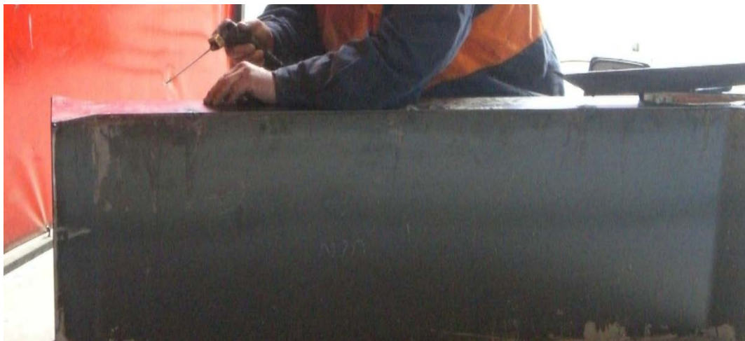
Figure 5.3: Welding of steel end cap to form a fully enclosed panel before testing.
