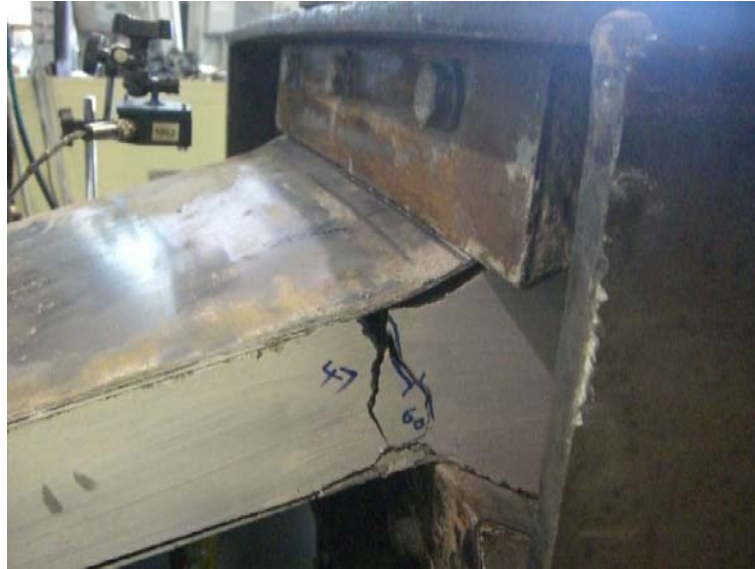
Figure 5.27: The flared end of the Control panel being pulled out from the keyed connection.
