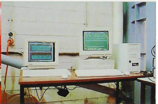
Figure 4.13 Data acquisition & control computers
