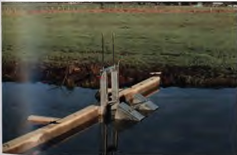
Plate 2.2: Self-Regulating Tilting Weir (built in 200 by UOW Acid Sulphate Soils Research Team)
