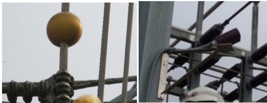
(b) The sphere (c) The pyrometer Figure 7. Pictures of the substation with the infrared thermometer and the sphere.
