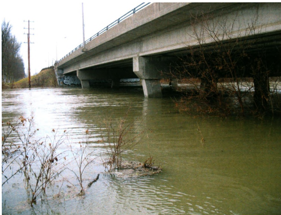
Figure 5.7: Flooding at Adelaide Street Bridge, January 2008 (Angela Peck, 2008)
