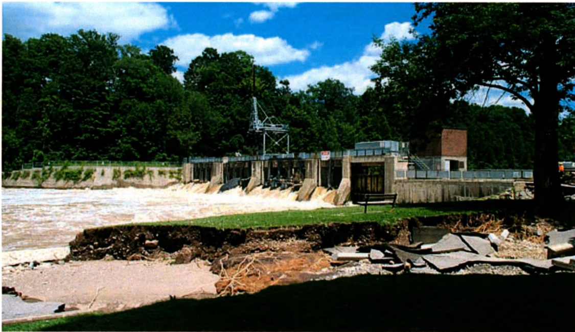
Figure 5.17: Road collapses at Springbank Dam in July, 2000 (UTRCA, 2000)
