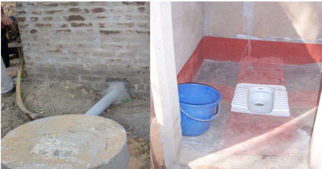
Figure 5.1. The faecal pit with concrete lid and inside of a pour flush latrine constructed as part of the Total sanitation campaign in Odisha, India.
