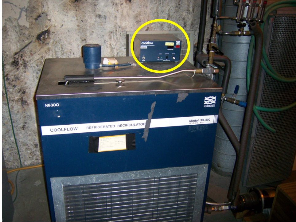
Figure A.5. Neslab recirculating chiller.
