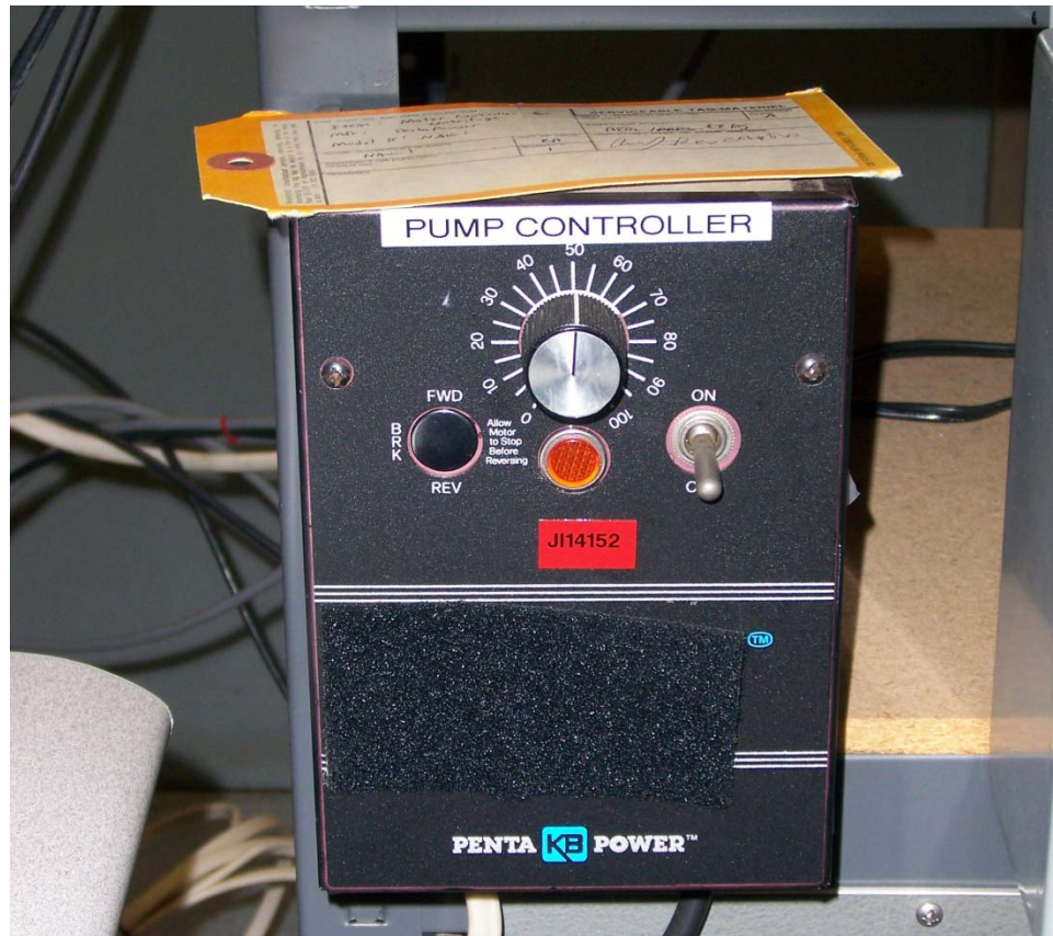
Figure A.7. Booster pump control panel.
