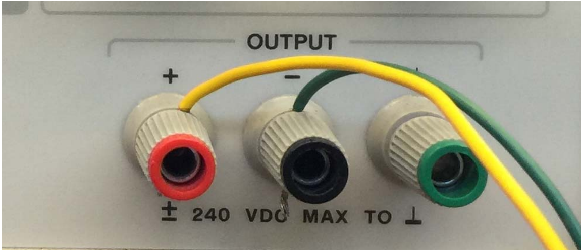
Figure 84. Speed control console to DC power supply connection.
