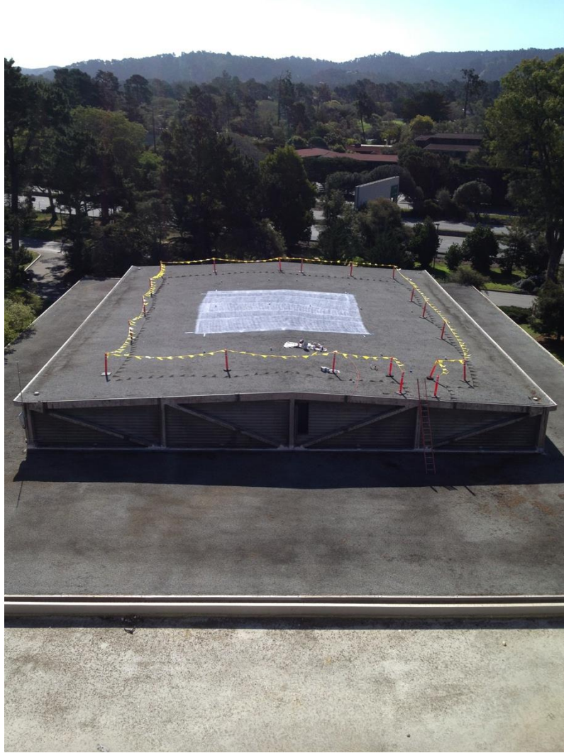
Figure 29. Safety setup atop King Hall showing the complete work area including visual safety barriers and entry point.
