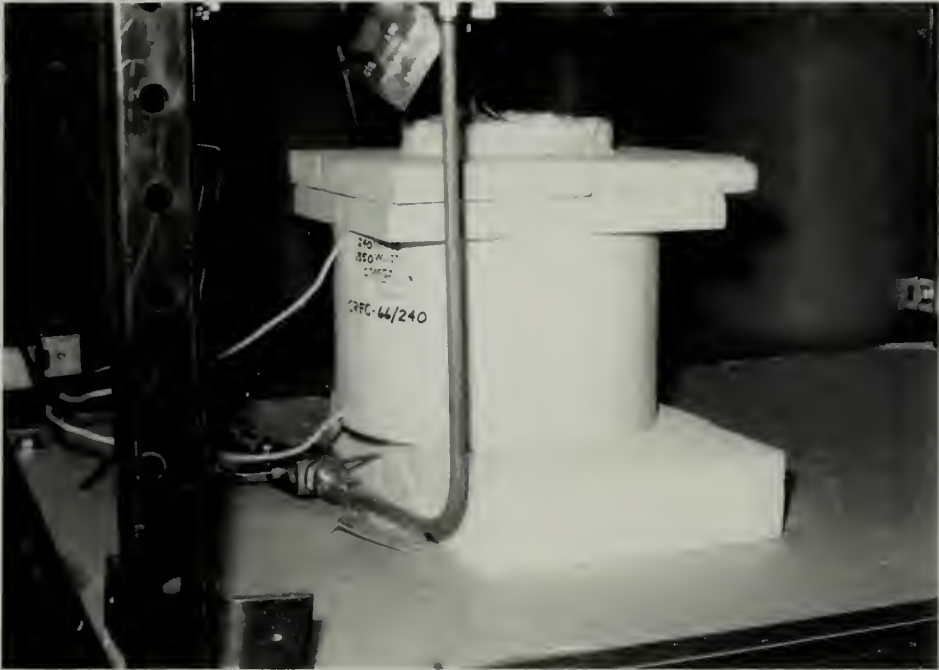
C-9 Preheater Heater and Partial Insulation
