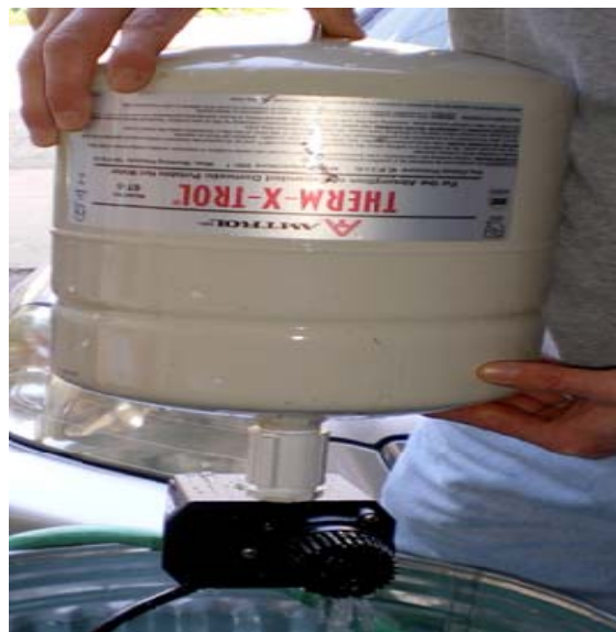
Figure 16. Submersible pump attached to expansion tank.
