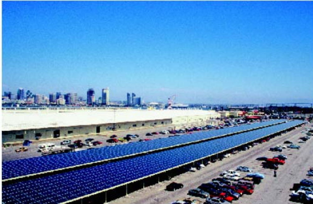
Figure 3. PV System at Coronado Base, CA
