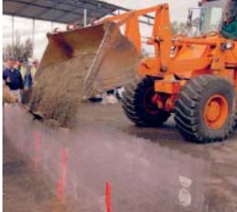
Figure 84. The Rapid Deployment Fortification Wall 345
