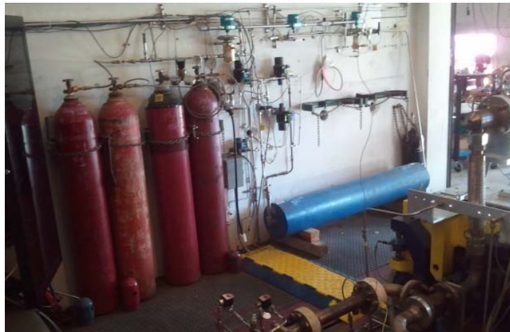
Figure 10. Test Cell 2 Fuel and Gas Tanks
