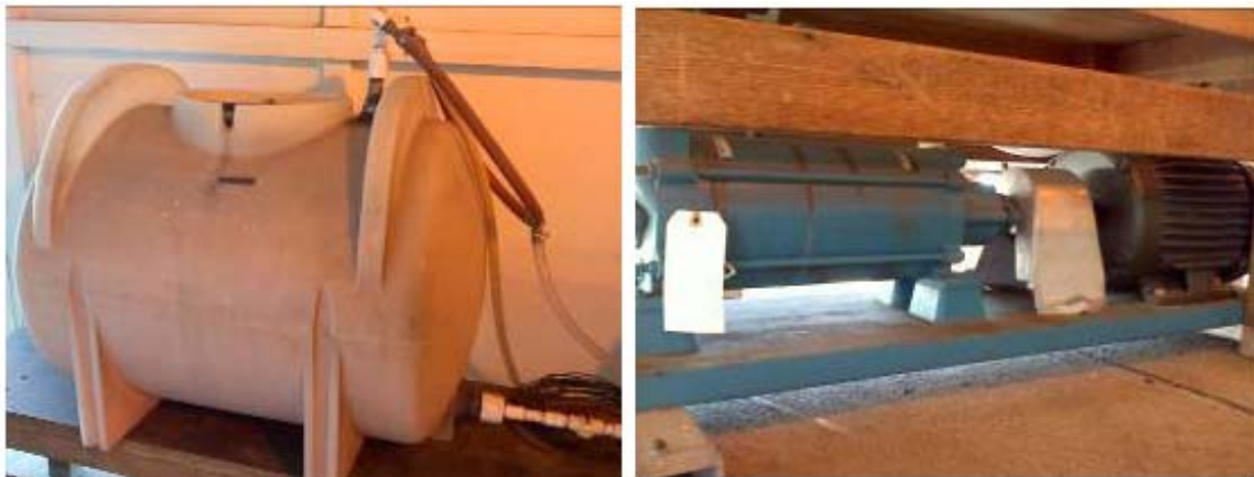
Figure 18. Cooling Water Tank (Left) and Regenerative Turbine Water Pump (Right) (From [8])
