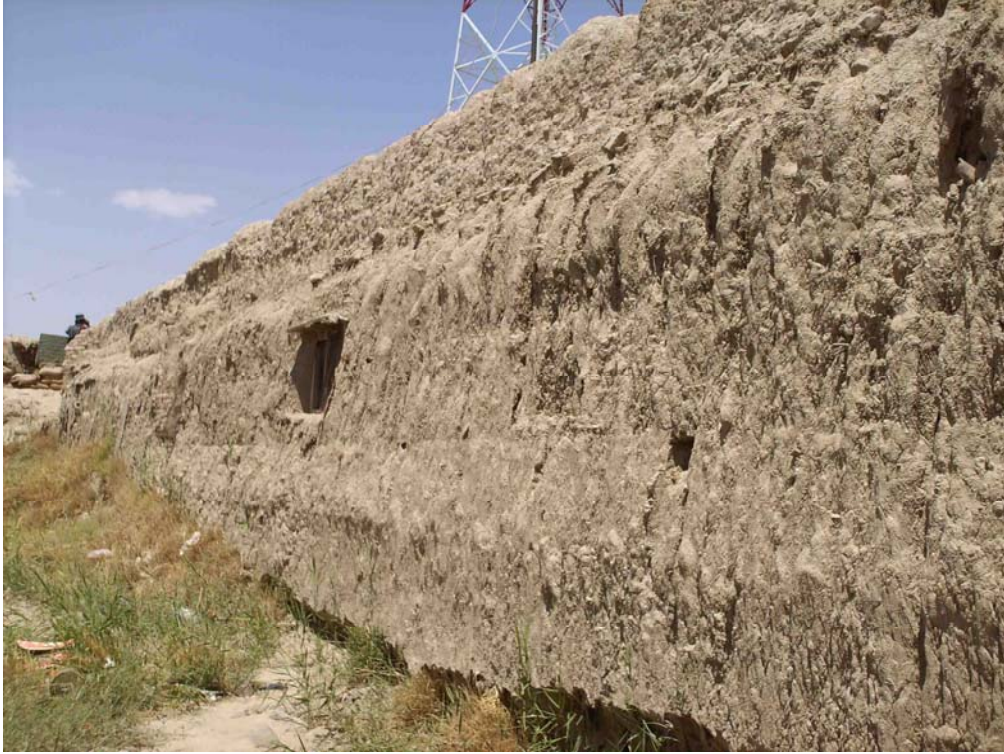
Photo 4. Erosion of Mud/Clay Mixture on a Clay Structure 298
