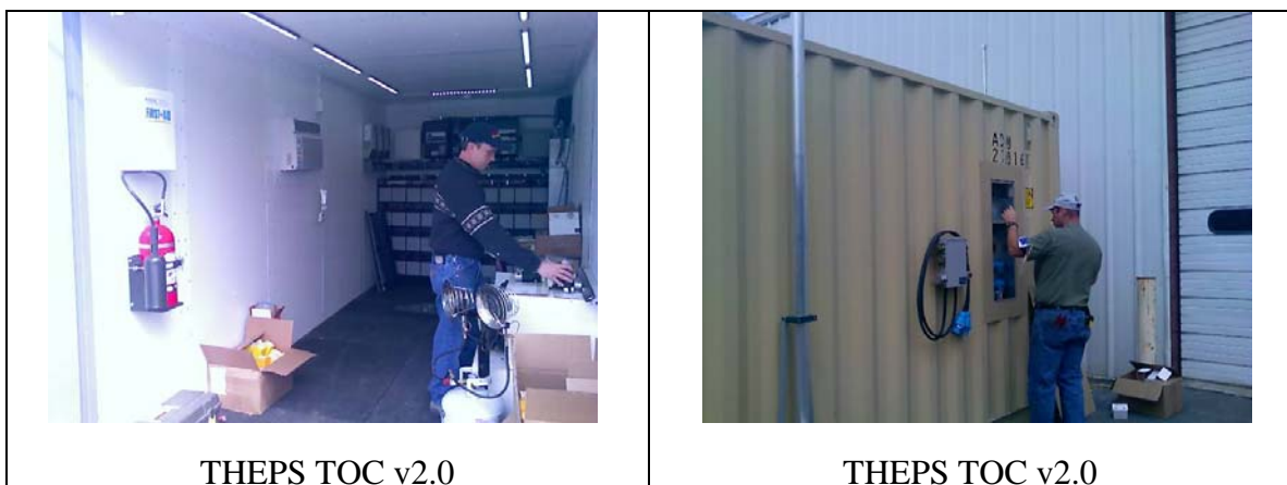
Figure 2. THEPS Variant Used as a Tactical Operations Center. From COL Dan Nolan, U.S. Army (Ret.) 2007.
