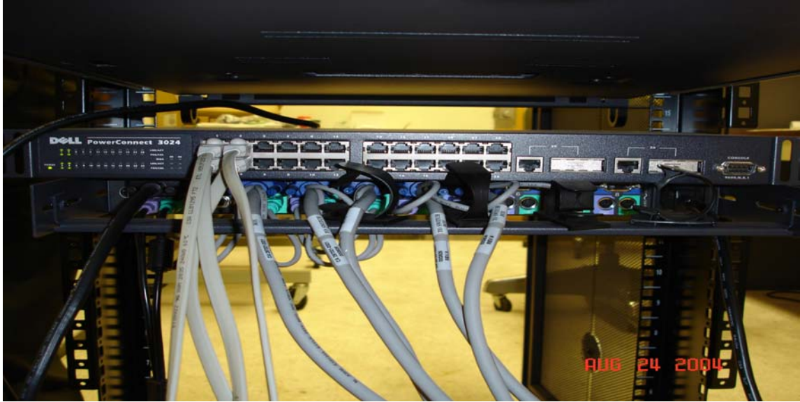
Figure 3. Dell PowerConnect 3024 Switch (top), and Dell 8 Port KVM Switch
