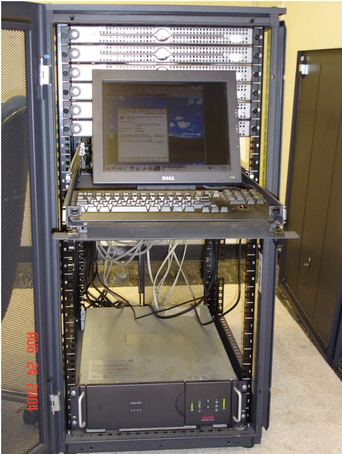
Figure 6. Dell PowerEdge 1650 Rack System
