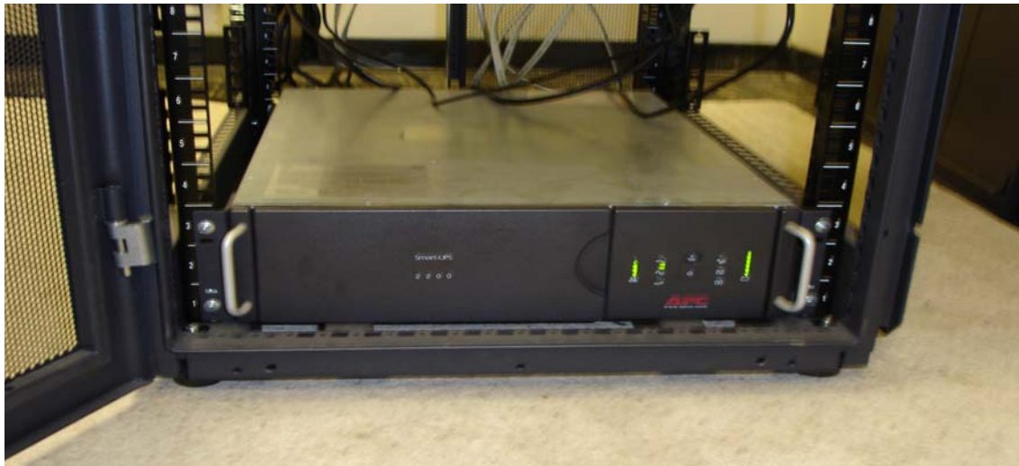
Figure 4. APC Smart UPS 2200 Power Supply
