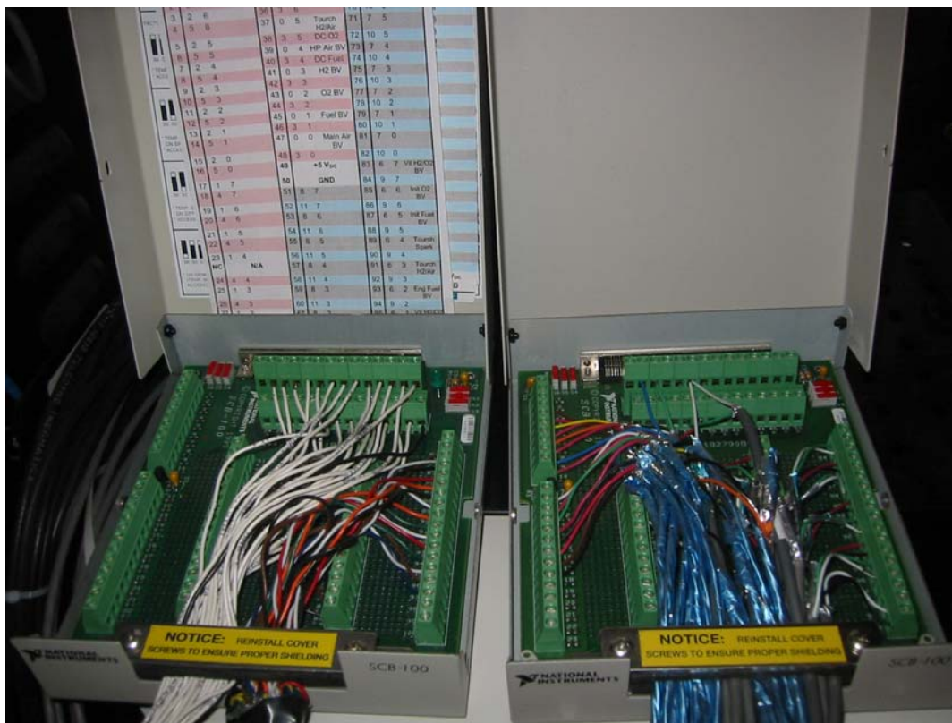
Figure 32. Breakout Panels for PXI 6508 and PXI 6031E Data Acquisition Boards
