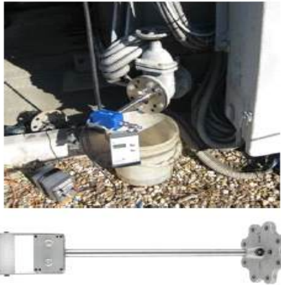
(a) Drain valve sensor
