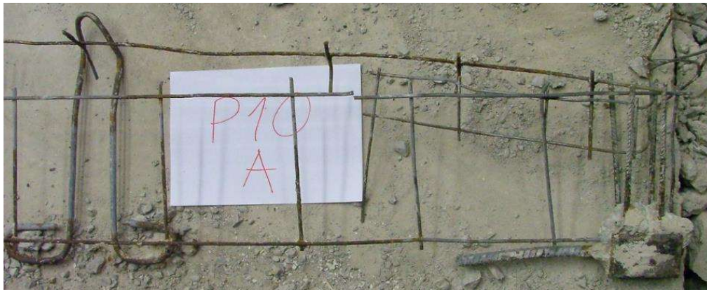
Figure 7. Photograph of the steel prestressing bar, reinforcements and eye bolt details of the longitudinal rib A-B of ribbed panel P10 (P10/A-B) after demolition.
