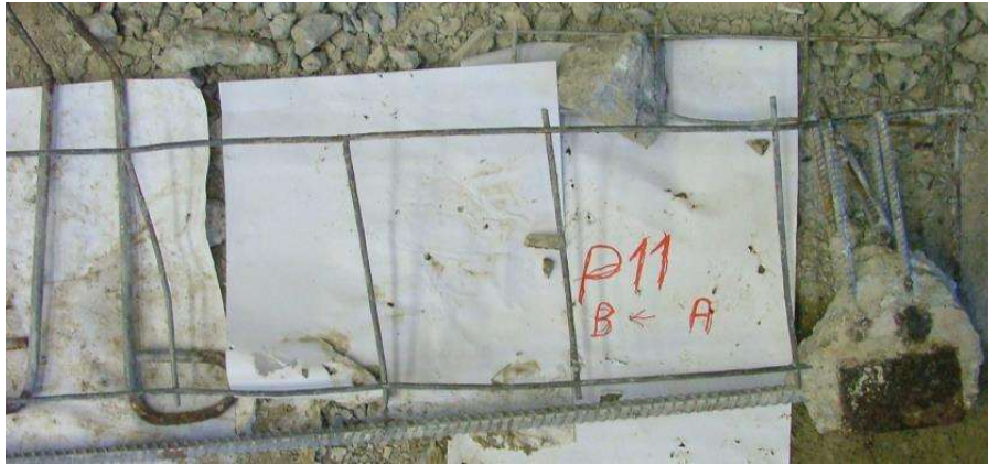
Figure 9. Photograph of the steel prestressing bar, reinforcements and eye bolt details of the longitudinal rib A-B of ribbed panel P11 (P11/A-B) after demolition.
