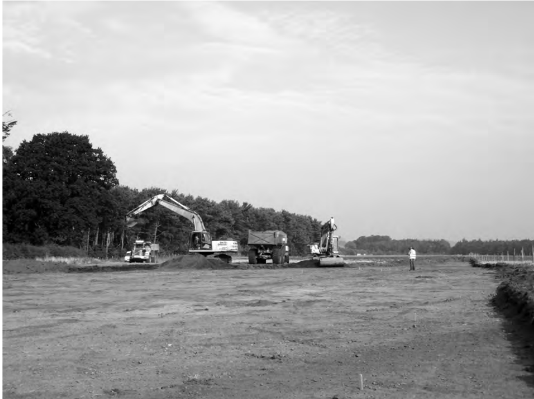
Fig. 7.13. The strip and record process underway at the Lanton Quarry site with features being catalogued and marked as they are revealed.
