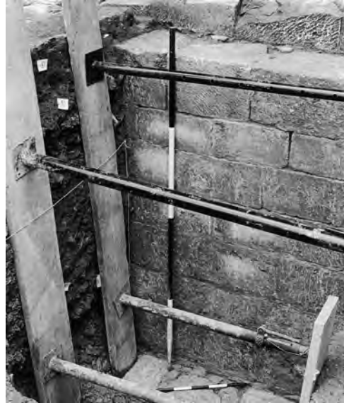
Fig 2.35 Looking south-east at the foundations cg101 of the retrochoir: lc84 Area A, LUB 1
